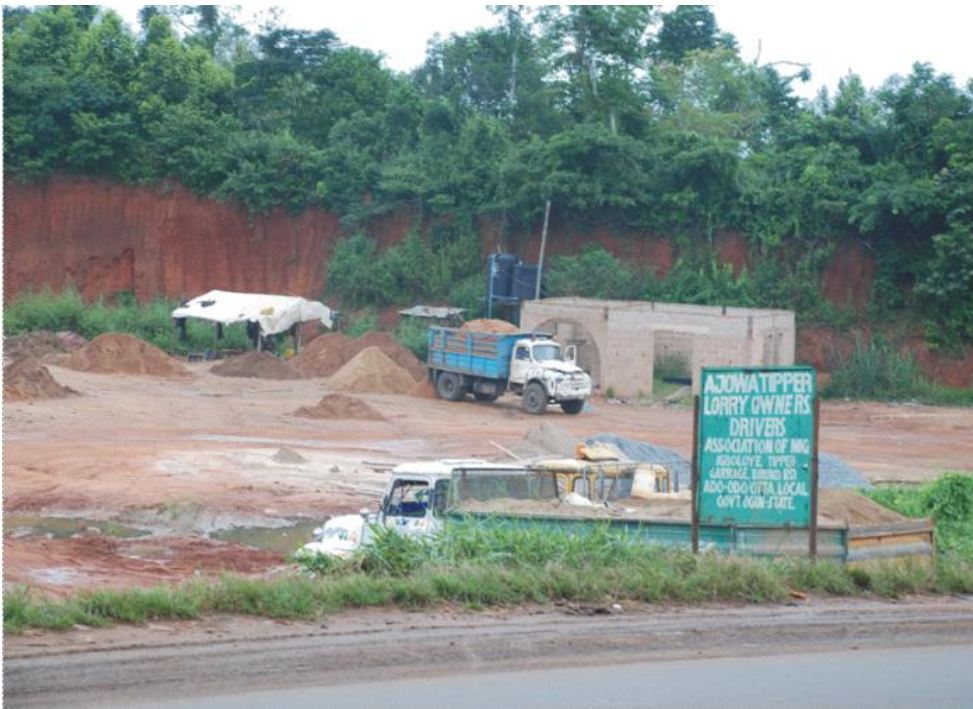
Plate 5: Depth of Excavation that Subsumes Vehicles very near the major Ota-Ildiroko international highway.
